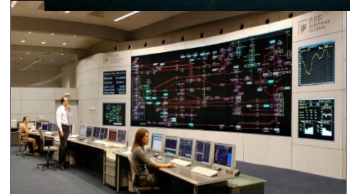
Wind energy in the control center
